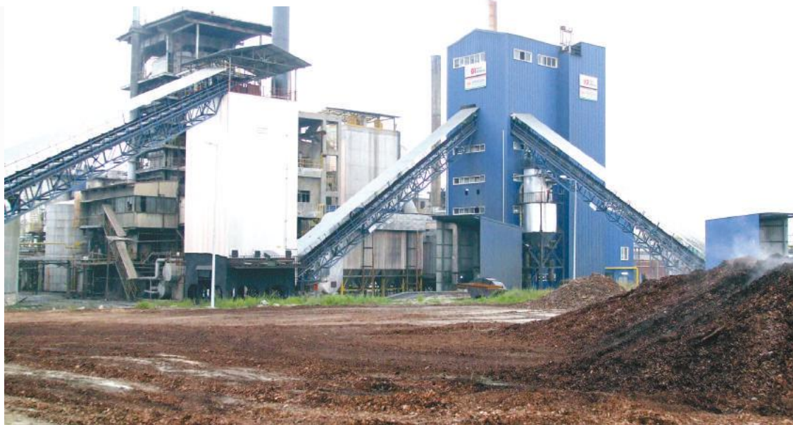
OYKA KAĞIT / ZONGULDAK 35 Ton/h 52 Barg 450 °C 4 MWe
